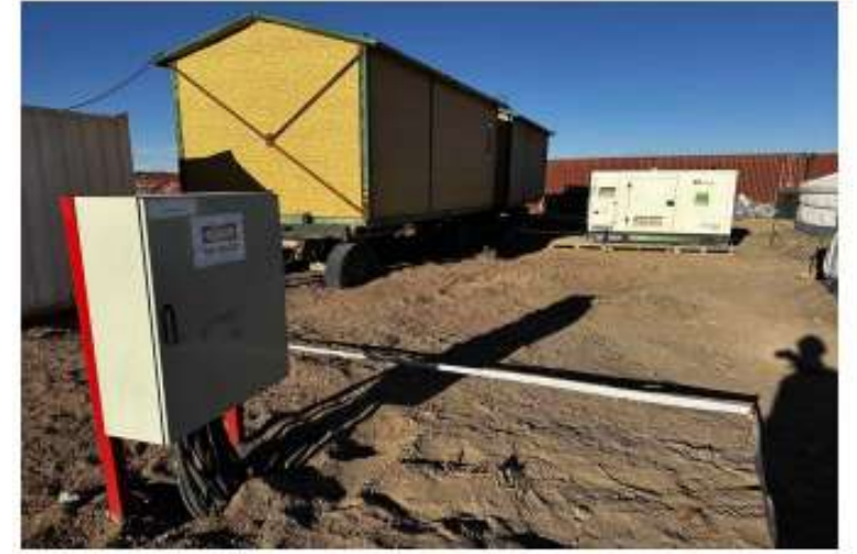
Ger Camp & Construction Power
