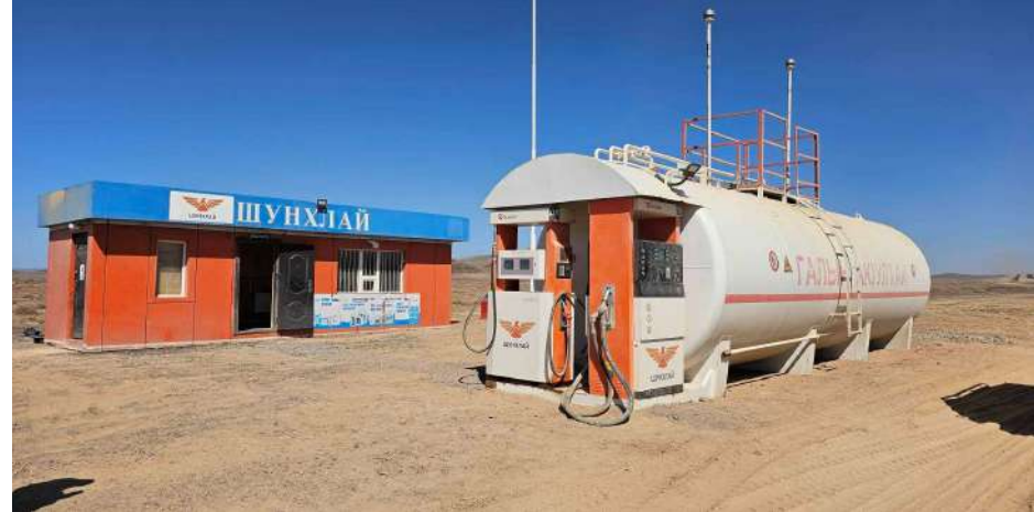
Temporary Fuel Station
