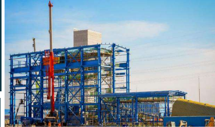
Oyu Tolgoi Underground Conveyor – MCS P
