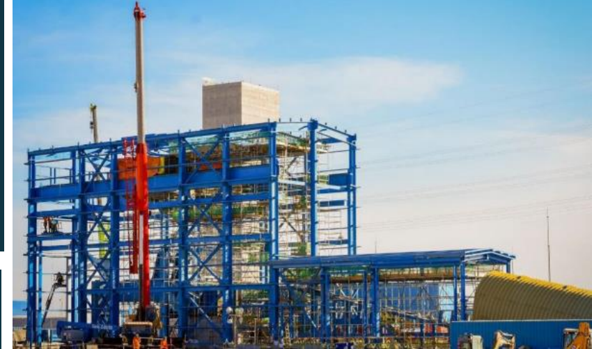
Oyu Tolgoi Underground Conveyor – MCS P
