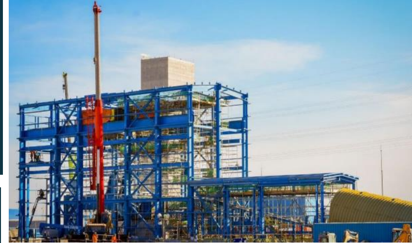
Oyu Tolgoi Underground Conveyor – MCSP
