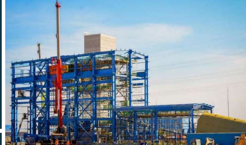
Oyu Tolgoi Underground Conveyor – MCSP
